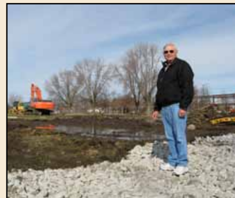
Jim Watkinson surveys the location of the new Hygienic Laboratory building prior to construction.
