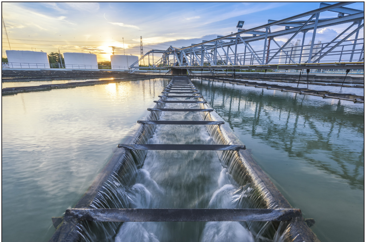
Wastewater treatment plant
